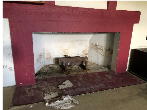
Photo M12 Woodburning Fireplace
