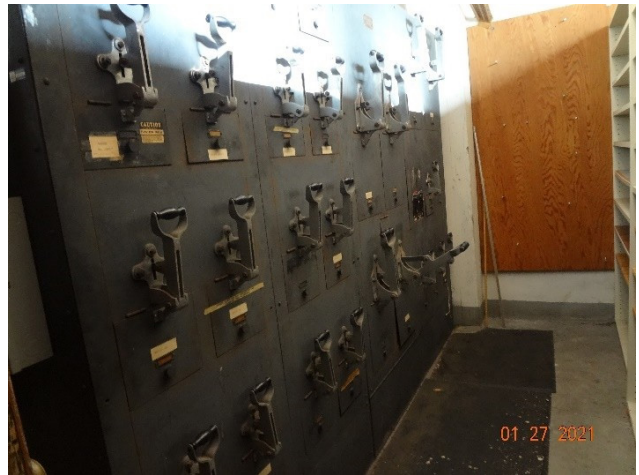
Photo E10 A panelboard may be built in late 1920's
