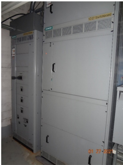
Photo E5 (2) Sections main switchboard
