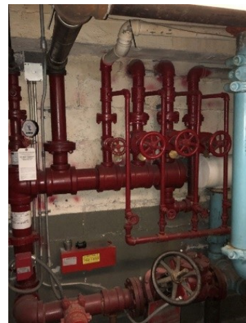
Photo FP2 Existing Fire Water Control Valves
