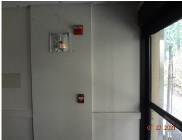
Photo E23 FA devices in infirmary building are in good condition.
