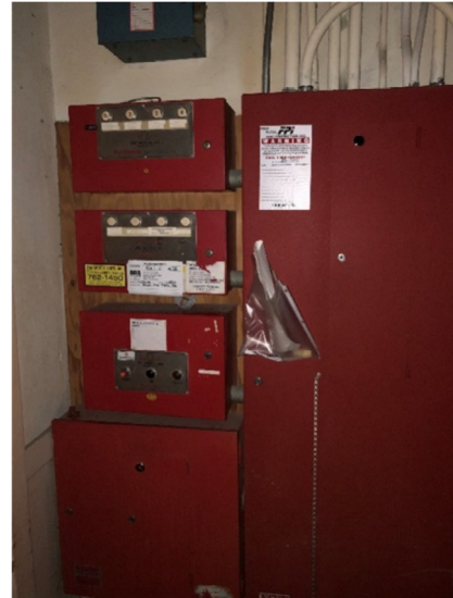
Photo E20 Fire alarm equipment in fair condition
