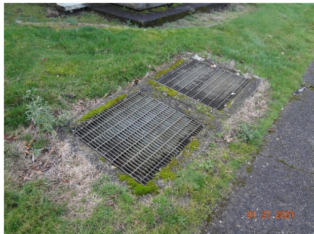
Photo E2 In-ground PSE vault
