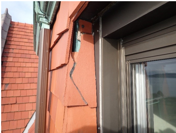
Photo BE9 Typical Terra Cotta Façade Damage
