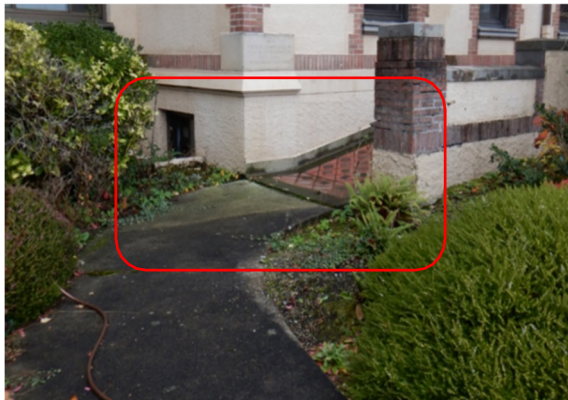
Photo ADA8 Access Ramp with Slope Greater than 1:12 and Rise Greater than 30 inches
