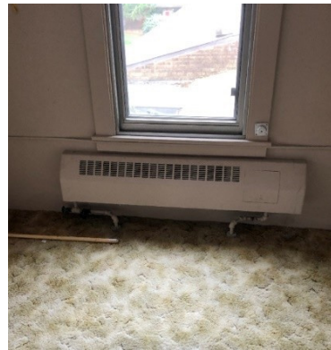
Photo M4 In-Room Radiator
