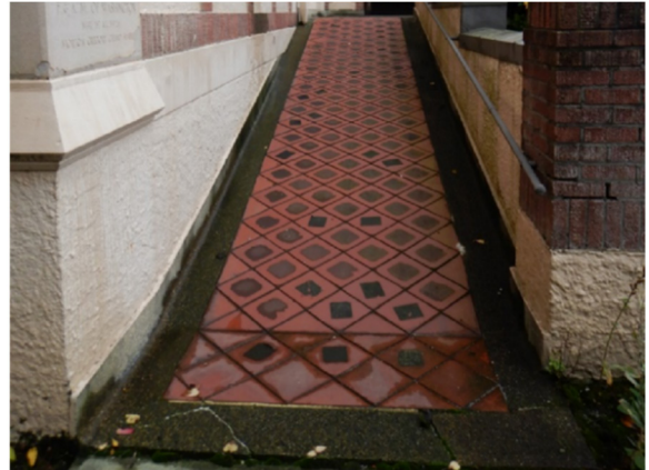
Photo ADA7 Access Route with No Landing at Bottom of Ramp
