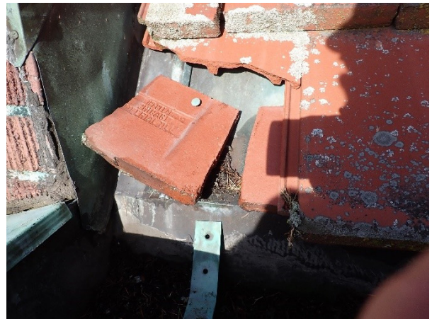
Photo BE10 Typical Terra Cotta Roof Damage
