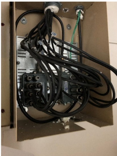
Photo E19 Cable terminal box in each floor janitor
