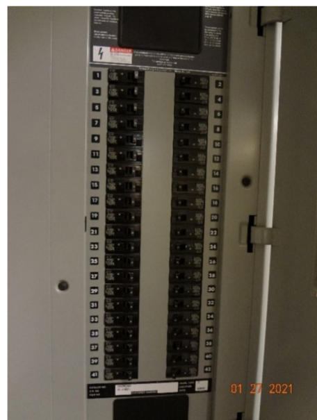
Photo E14 Panelboards in infirmary building in good condition
