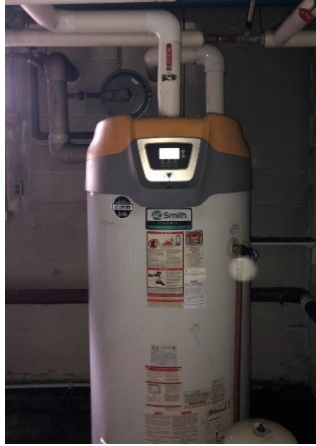
Photo P1 Existing Water Heater
