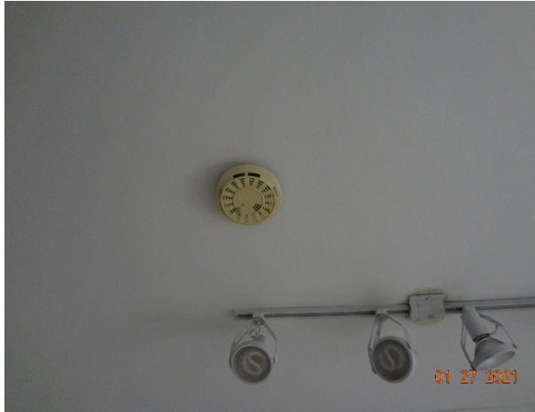
Photo E21 FA devices are outdated
