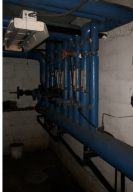
Photo M9 Heating Water Distribution Manifold
