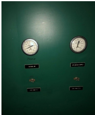
Photo M3 Pneumatic Controls
