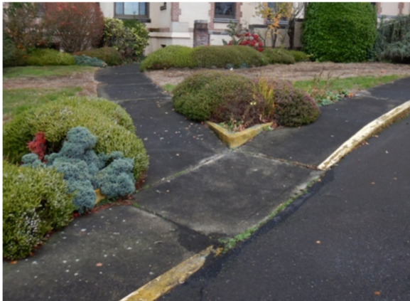
Photo ADA6 Access Route Walkway Surface with Slope Greater than 1:20
