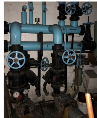
Photo M8 Heating Water Pumps and Distribution
