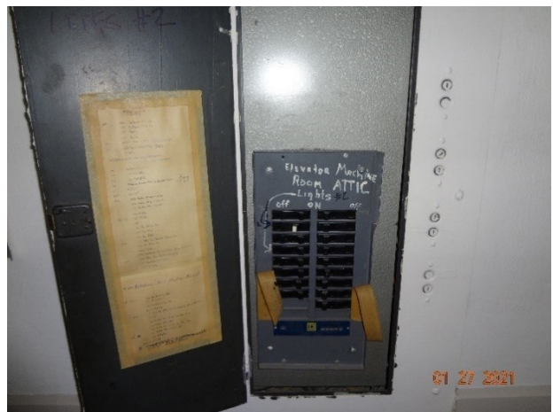
Photo E12 Panelboard in working but poor condition
