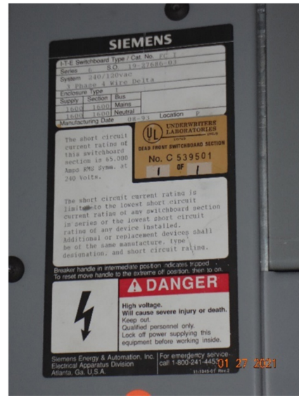
Photo E6 Main switchboard rating tag
