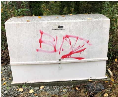
Photo P3 Hot Box for Domestic Backflow Preventer
