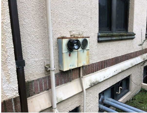
Photo E3 PSE meter exterior wall mounted
