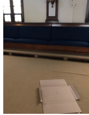
Photo M10 Under seat Ventilation within Hall
