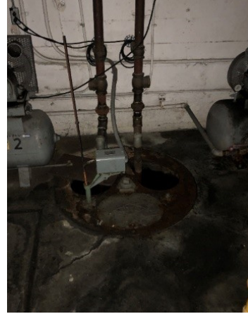
Photo P2 Existing Sump Pump
