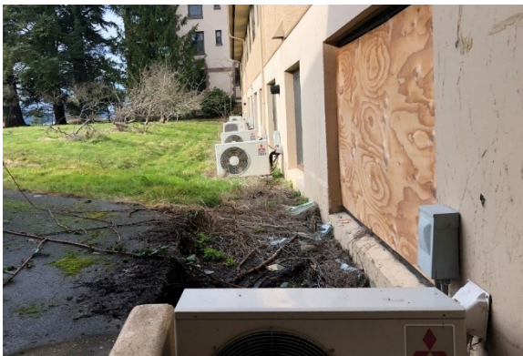
Photo M5 Split System Heat Pumps
