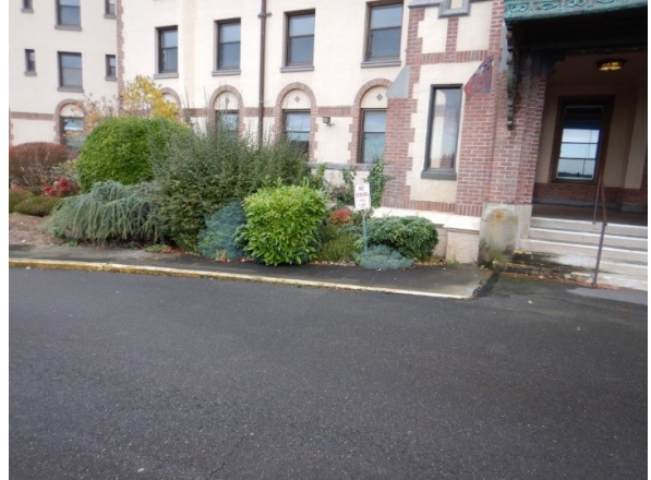
Photo ADA5 Overgrown Shrubbery in Access Walkway
