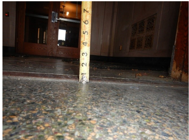
Photo ADA15 Main Entry Threshold Height, ≤1/2 inches
