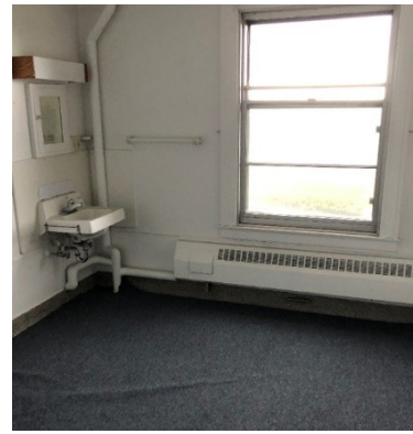
Photo P4 Dwelling Unit Plumbing
