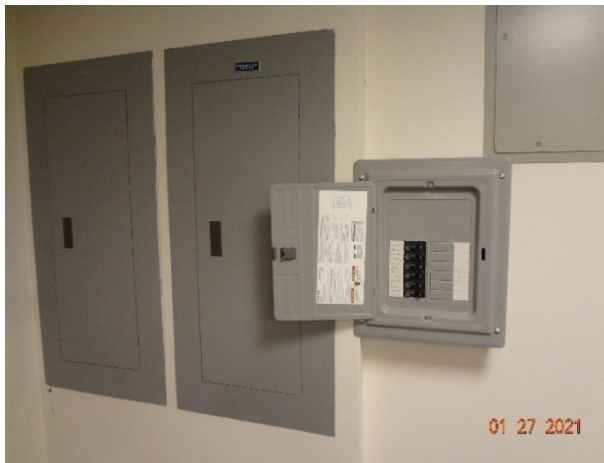
Photo E13 Panelboards in infirmary building in good condition
