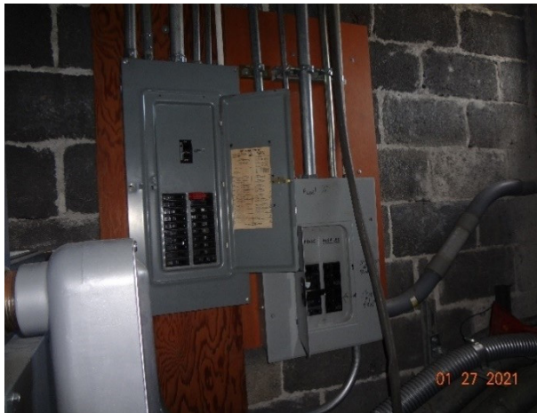
Photo E11 Panelboards may be upgraded with main switchboard in mid-1990's
