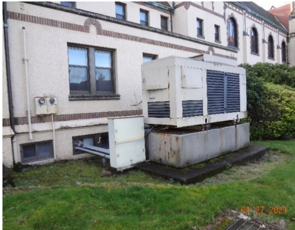
Photo E9 Generator sit outside building
