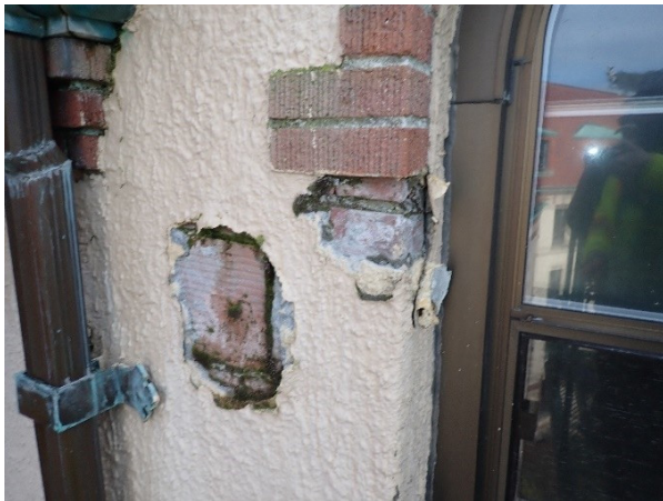
Photo BE3 Typical Wall Plaster Damage
