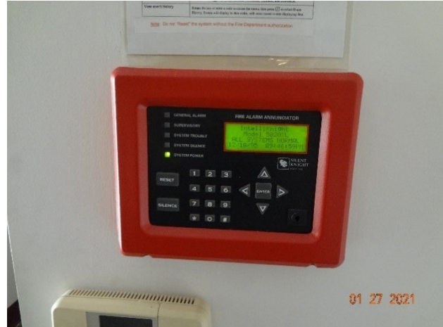
Photo E22 FA annunciator in infirmary building is in good condition
