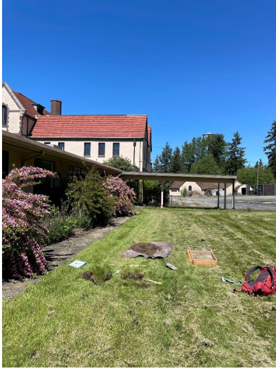
Figure 6-3. Overview of proposed demolition area on the east side of the main building (view north).
