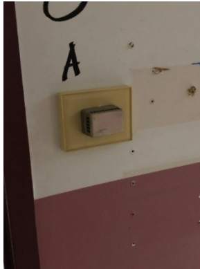
Photo M11 Pneumatic Thermostat
