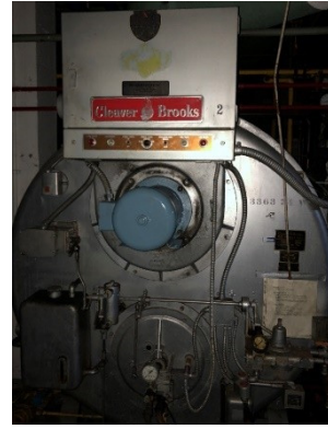
Photo M2 Abandoned Boiler #2 (3 is Similar)
